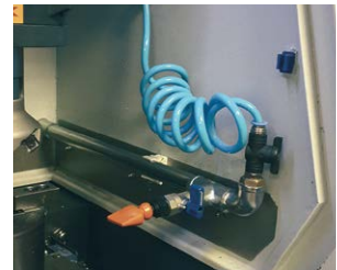
Air Cooling System
